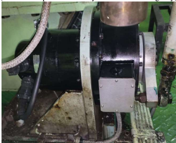
(An actuator painted black by an unauthorized agency)
